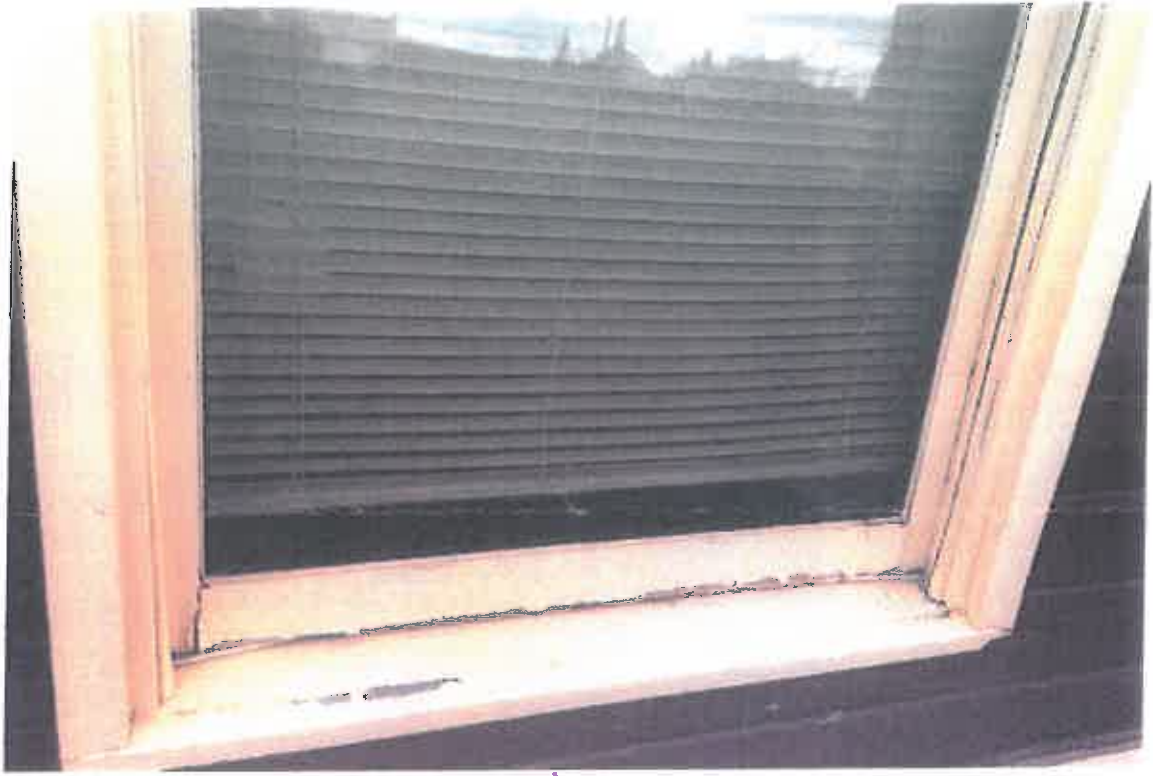
Rotten window frames
